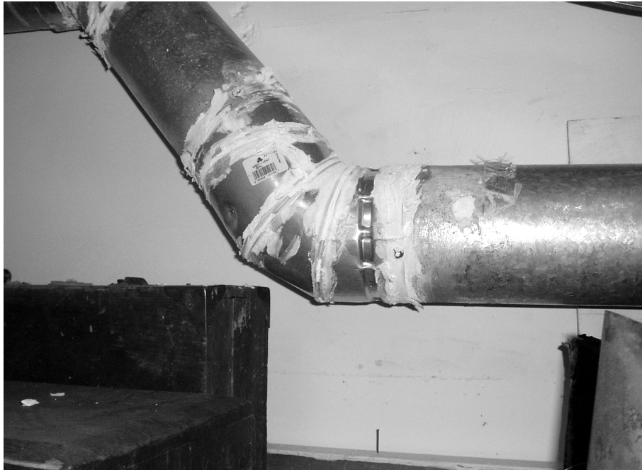
Collections Storage – exhaust duct over storage shelves exiting west wall – a nasty item to have in the collection room. Photo by author.
