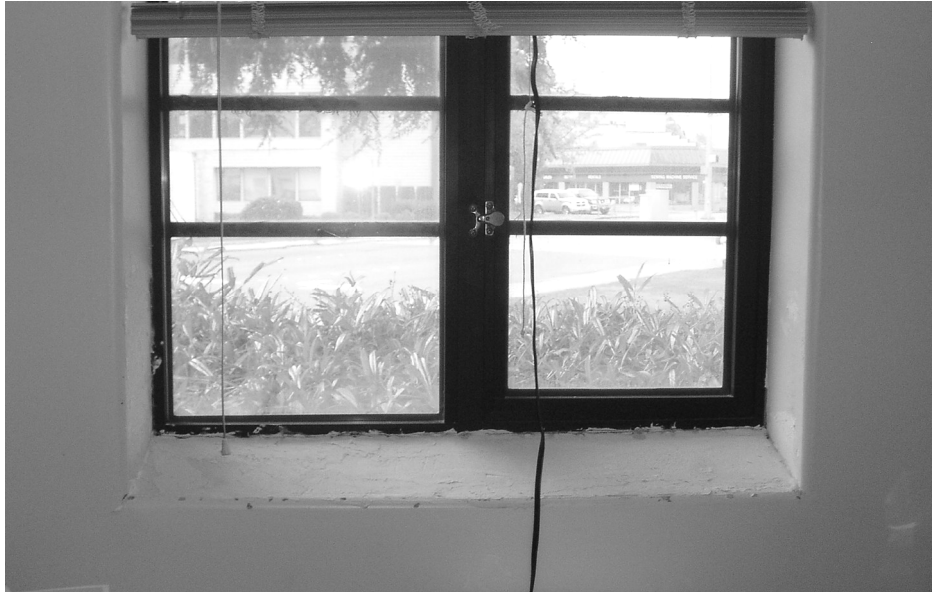
Window at workroom, typical, showing spalling finish at window surround. Photo by author.
