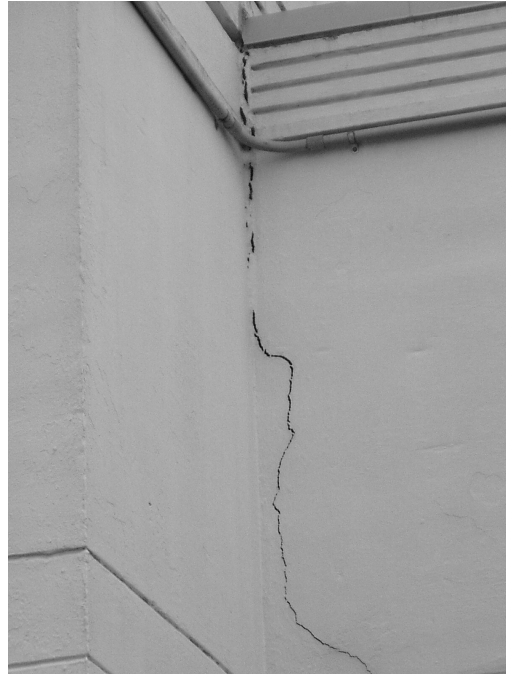
Crack at wall, 2007. Hose tower at left. Photo by author.
