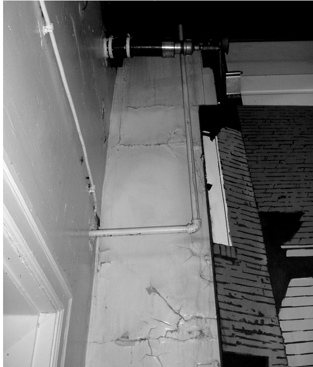
Efflorescence at west wall near overhead door causing paint to blister & crack. Photo by author.
